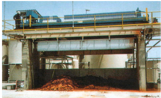
2m x 1.5m Filter Press (Gold Mine)
